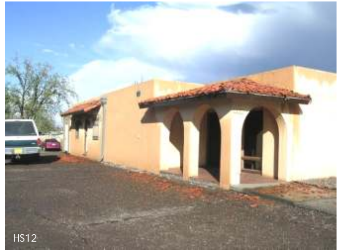
Homes and buildings with tile roofing were severely damaged – this is a local dentist's office about a mile southwest of the AOC.
