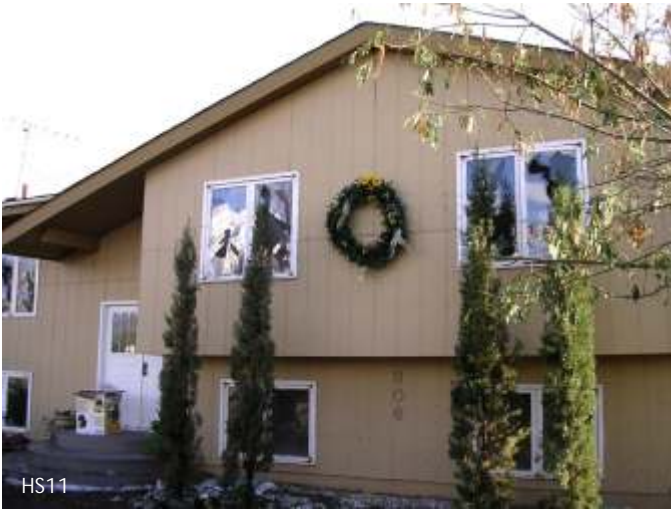
Typical house damage. Many north and west facing windows were broken. The hailstones passed through the triple-paned windows on this home.
