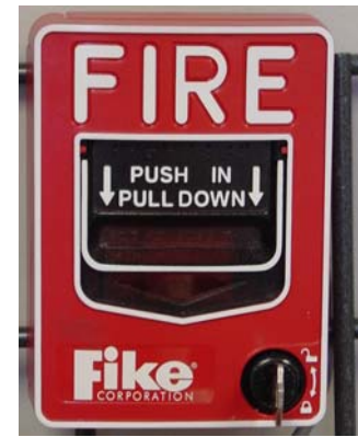
Exhibit 3-40 Addressable Pull Station
